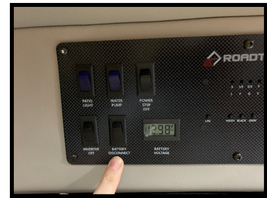
Picture 40.3 Battery disconnect switch
