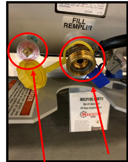
Propane bleed valve and propane fill valve
