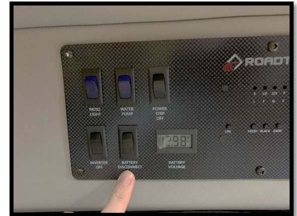
Picture 37.1 Battery disconnect switch
