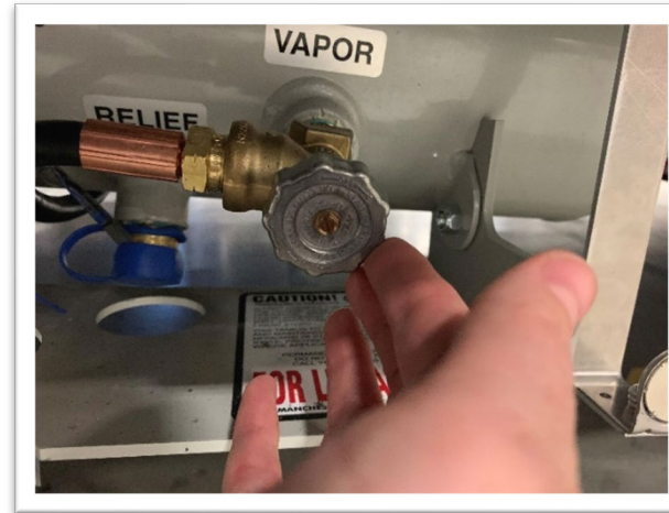
Propane tank main shutoff valve
