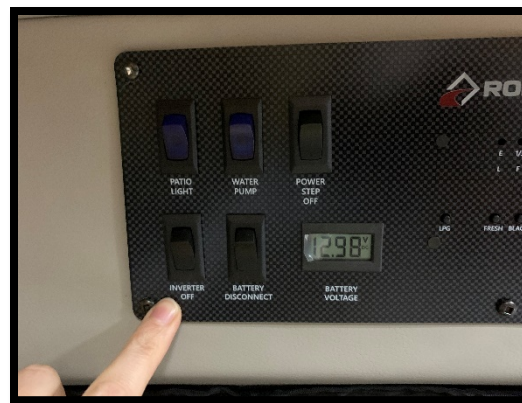
Picture 40.2 Inverter switch
