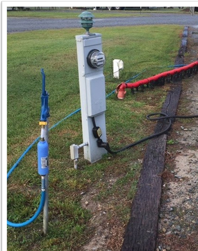
Full hookups - electric, water, and sewer
