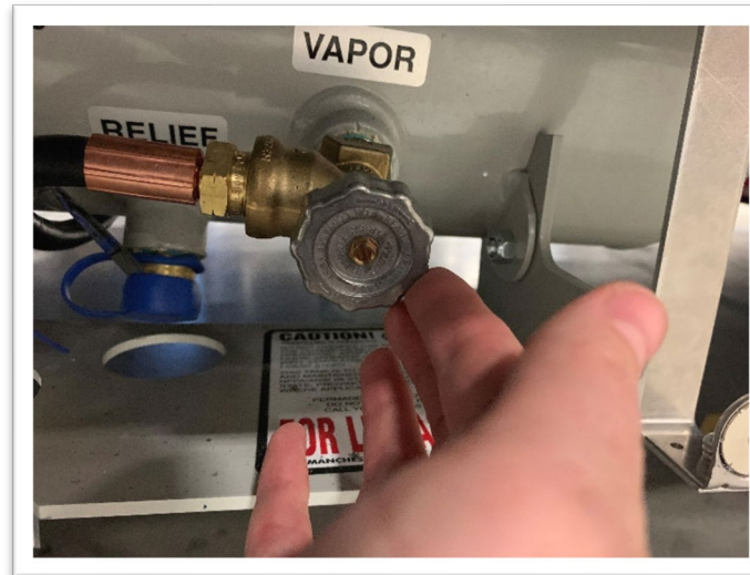
Propane tank main shutoff valve
