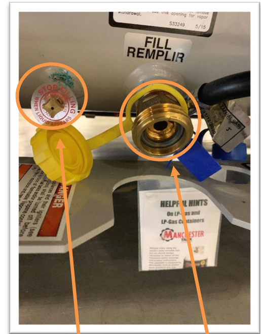
Propane bleed valve and propane fill valve
